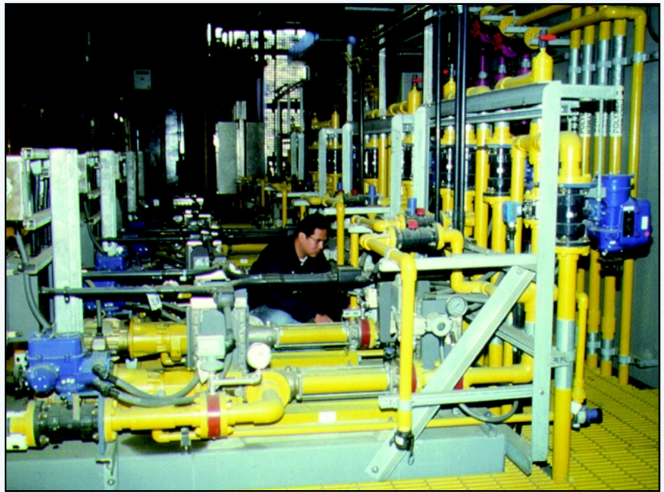
Photo 2. Author Ernie Molas inspects progressive cavity polymer feed pumps (foreground) used to transfer to thickening centrifuges. Additional PC units (rear) move thickened sludge through a screening system to blending tanks.
