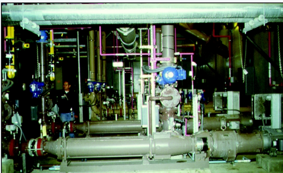
Photo 1. Progressive cavity sludge pumps feed thickening centrifuges at up to 1,000 gpm.
